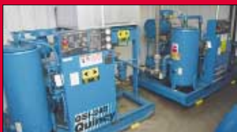
Bank View 100 HP and 50 HP Quincy Air Compressor
