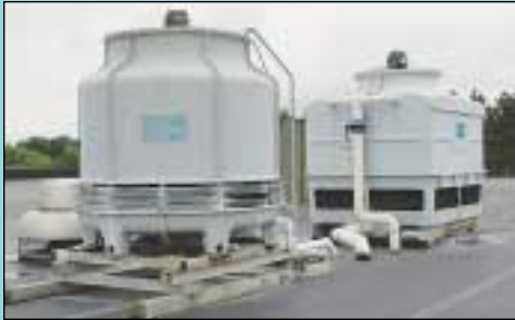
(2) Thermal Care Fiberglass Cooling Tower Cells
