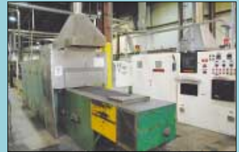
(2) 12" Wide CI Hayes Type BACM-ACL Continuous Mesh Belt Electric Fired Heat Treat Furnaces
