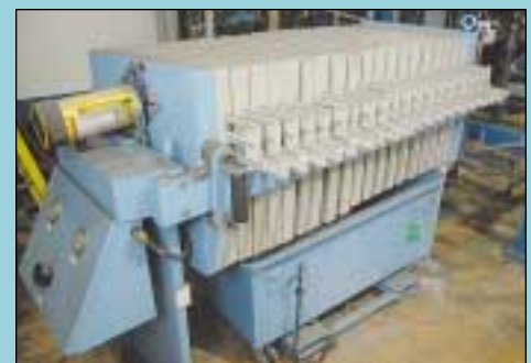
Waste Water Treatment System - Filter Press View
