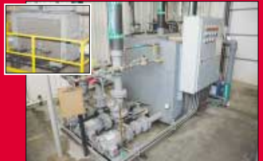
Partial View Late Model Chiller and Cooling Tower Systems
